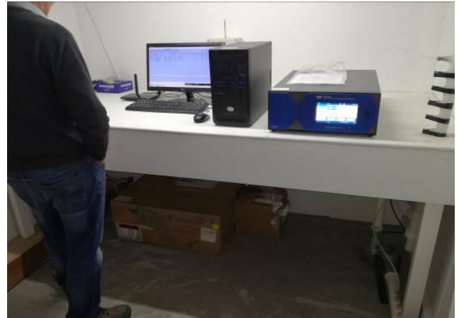
Air Quality Monitoring equipment installed in Velddrif
