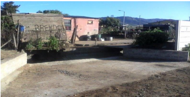
Stormwater channel automatic overflow
