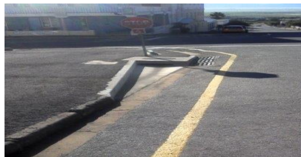
Newly design storm water inlets in steep areas
