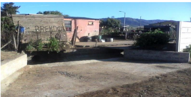
Storm water channel automatic overflow
