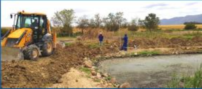
Upgrades to the Waste Water Treatment Works in Porterville is well underway
