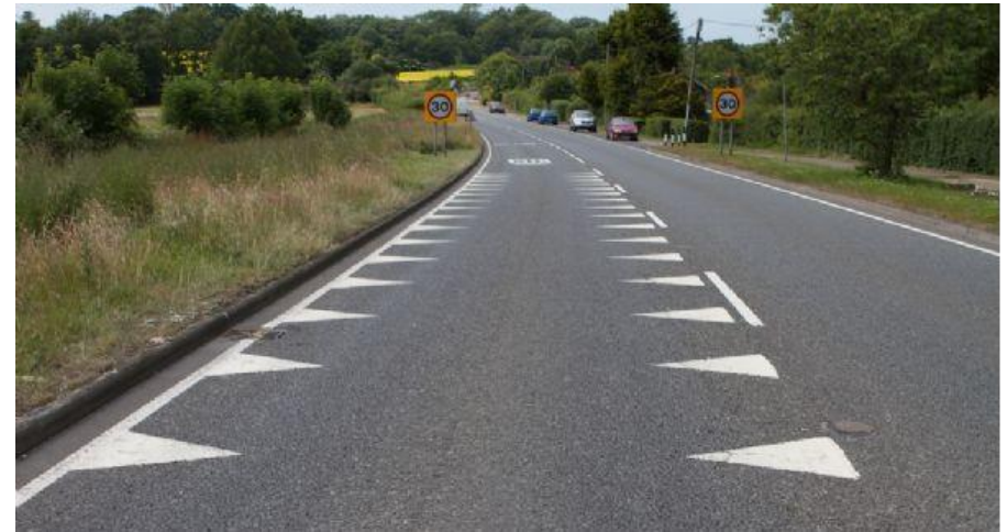
Image 30: Road markings on major throughfare roads result in slower moving vehicles, which can in turn lead to motorists taking more interest in their surroundings
