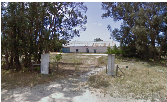
FIGURE 41. A DEGRADING OLD BARN ALONG VOORTREKKER ROAD
