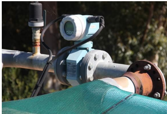
Endress & Hauser bulk raw water meter for Aurora
