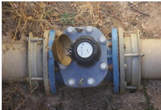
Bulk water meter on inlet of 2.4 MI Piketberg reservoir
