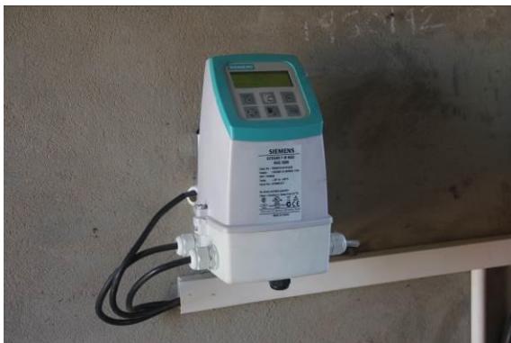
Siemens bulk water meter for Porterville WTW
