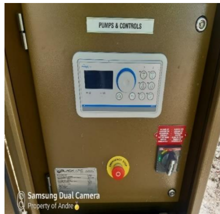
New MCC panels installed at pump stations
