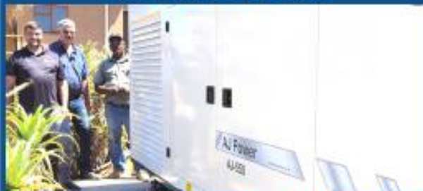
Bergrivier Municipality was awarded R3,4 million from the Western Cape Government which was used towards purchasing two large generators (550kWh and 330kWh) to ensure sufficient water purification for Piketberg.
