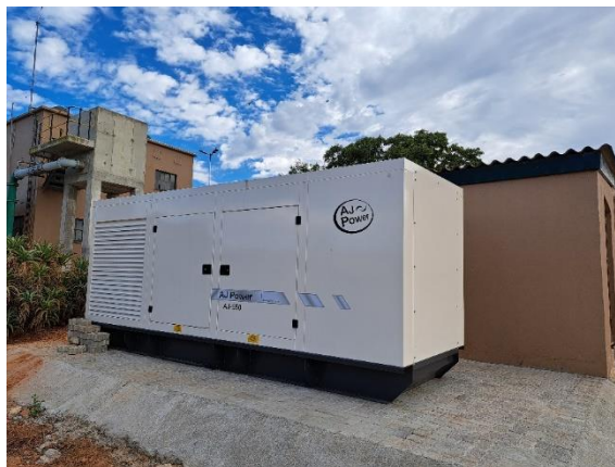
550Kva generator installed at Piketberg Water Treatment Works
