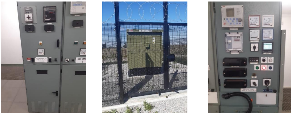
Images above (from left to right): Noordhoek Substation, New Port Owen Ring Main Unit (RMU), Port Owen integrated into main feeder.
