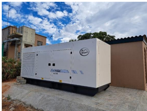
550Kva generator installed at Piketberg Water Treatment Works
