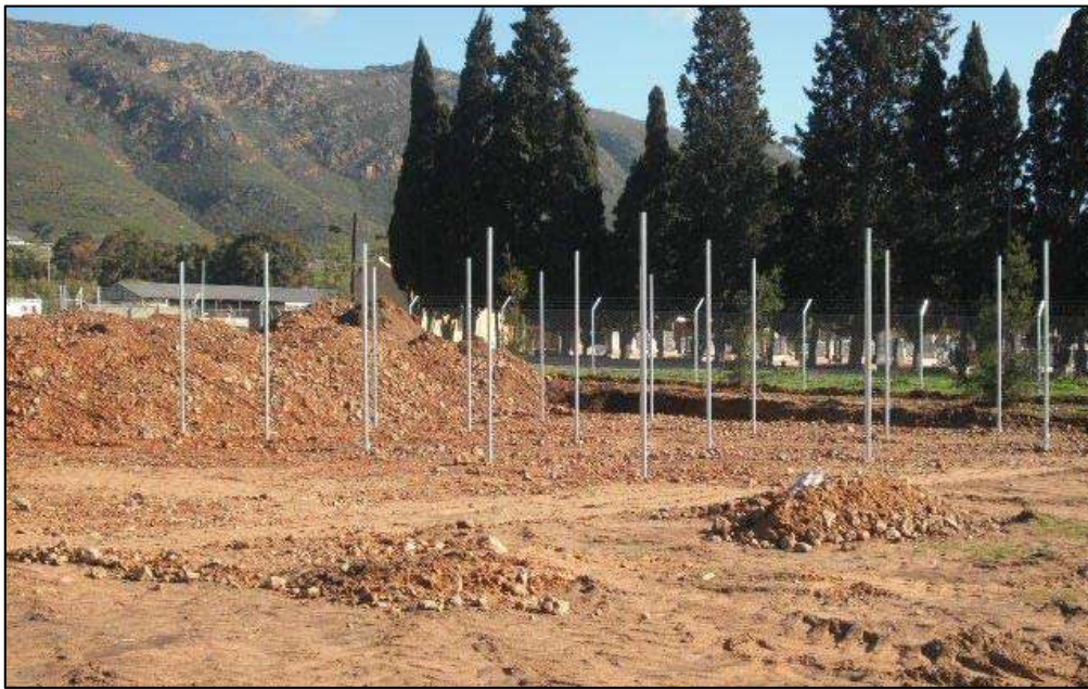
Construction of new cricket nets at Piketberg Cricket Nets Photographer unknown: Photo provided
