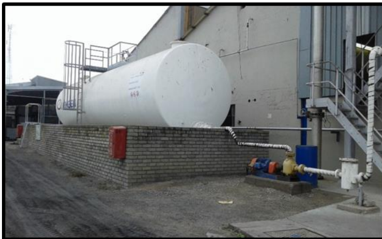
Bulk fuel storage at Amawandle Fish Factory Laaiplek
