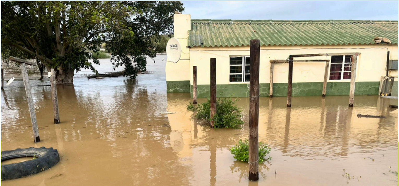
Adverse weather: The Western Cape experienced extreme weather in the form of heavy rainfall, damaging wind speeds, severe flooding and lots of destruction of infrastructure. Bergrivier Municipality was no exception and had to face two weeks of disruptive rainfall and high wind speeds causing extensive damage to public and private infrastructure, and the need arose for the activation of a Joint Operation Centre to provide relief to affected residents. Photo: Moravia Area
